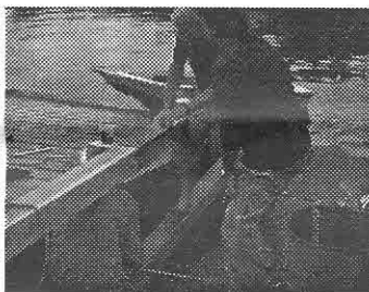
John DiLallo, Peter Broecker and Laurence Concannon (under dock) install new sides on the dinghy-launching ramp
